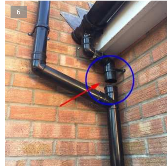
Downpipe has dropped away from joint. Requires lifting back into joint and refixing. Additional bracket recommended to support weight. 05/02/2021 10:29 (GMT) at 52.13128277571139°, -0.012191729620110421°
