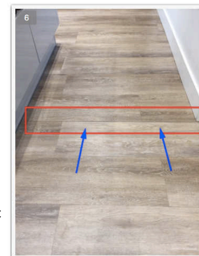
View of kitchen floor, existing floor into solid concrete extension floor. Uneven joint observed, gap in covering.
